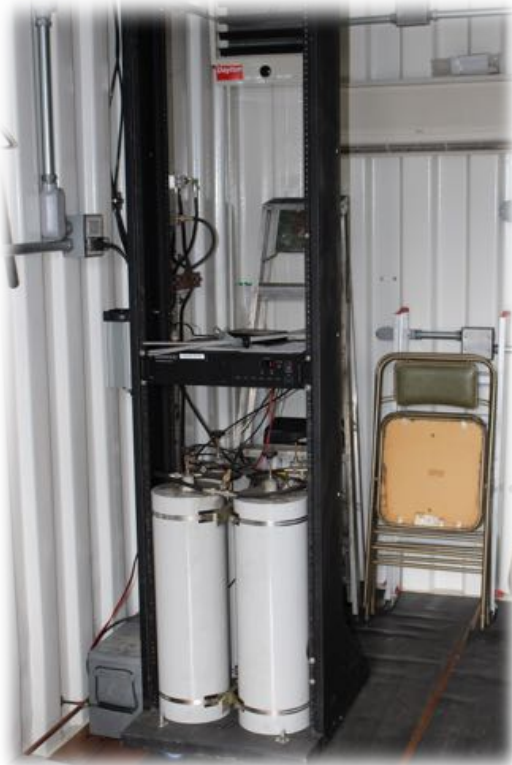
Repeater in its new rack.
